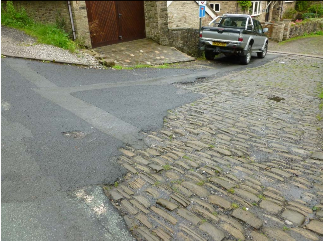
Setts at the entrance to Holly Vale & the intrusion of a modern road surface
